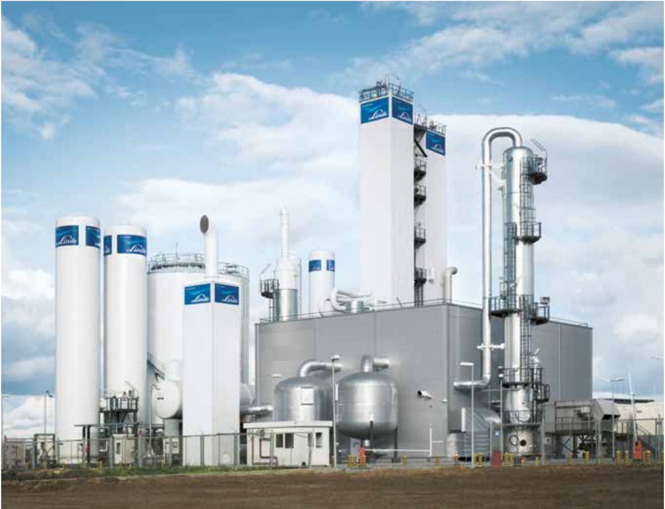
A LINDE AIR SEPARATION PLANT FOR ON-SITE SUPPLY OF AIR GASES INCLUDING OXYGEN, NITROGEN AND ARGON TO A MAJOR STEELWORKS IN RUSSIA.
