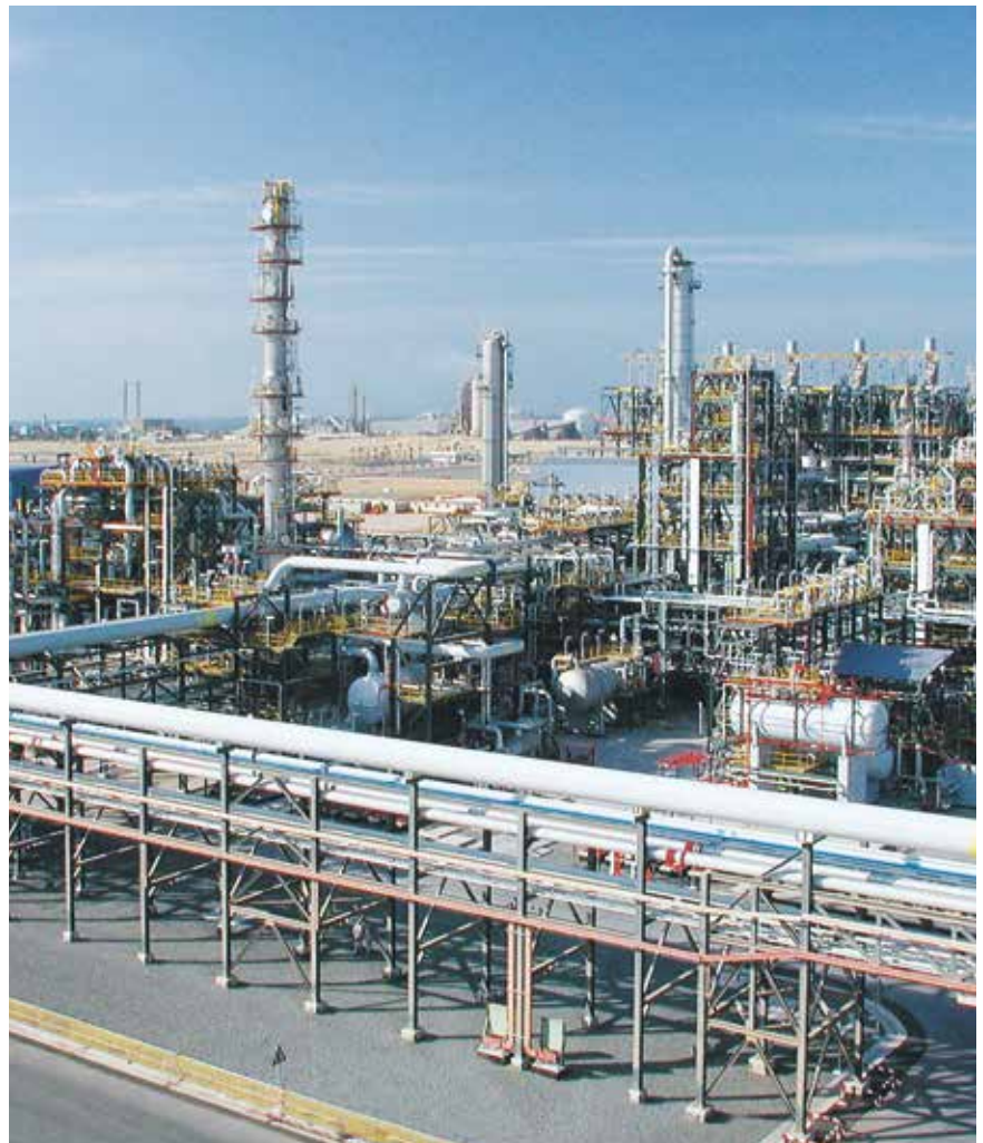
ETHYLENE PLANT CONSTRUCTED BY LINDE FOR A PETROCHEMICAL CUSTOMER IN RUWAI, ABU DHABI.
